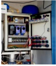
Figure 6: Electrical equipment box
