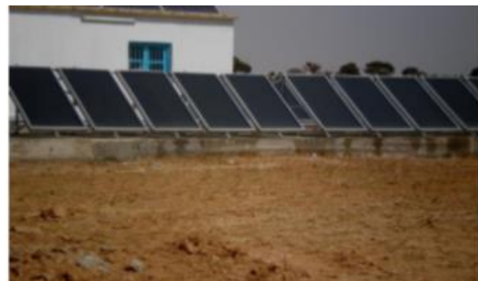
Figure 3: Field of solar collector thermal
